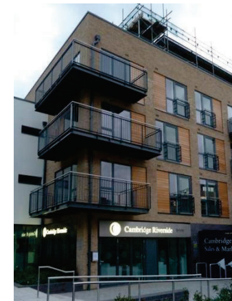
Extensive stained weatherboards at Cambridge Riverside devt
